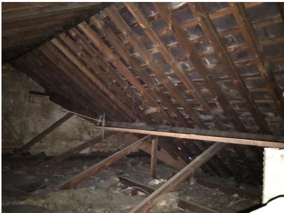
Internal loft space –Un-felted, evidence of water ingress can be seen to the underside of slate perp joints, showing angle of creep and calcification of slates. Evidence of water staining can be seen on purlin.
