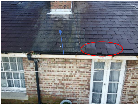
Insufficient or no fixings used to install, no evidence of nails being used through slates. Evidence of High water Absorbency below the chimney stack. Which would indicate slates are approaching the end of their useful life.
