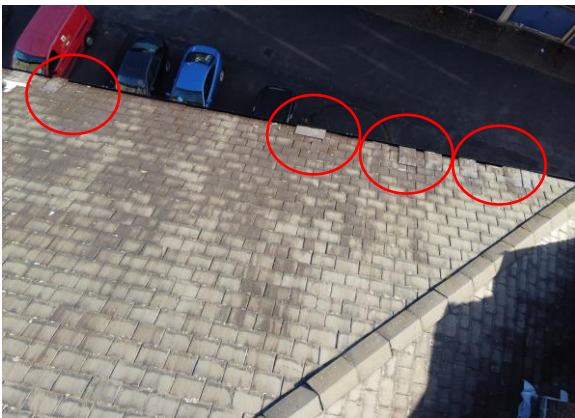
Evidence of Slate slippage on eaves course presenting a Health and Safety concern for the pedestrians at street level.
