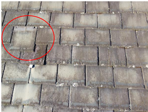
High levels of calcification evident from whitening on surface, geological symptoms of a softening slate. Further slate slippage
