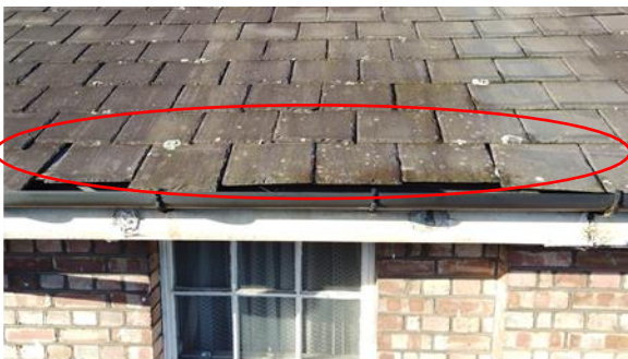
Noticeable slant on the eaves course perhaps caused by water ingress to the internal roof structure and swelling of roof structures. Evidence of top edge of fascia board rotting hence drop in eaves course.
