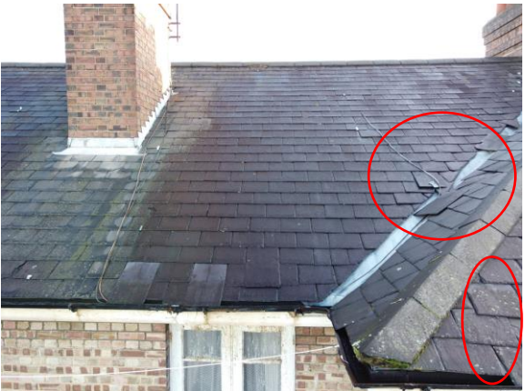
Evidence of loosening of slates due to wind damage, and possible vortex on leeward side of hip and leading to failure of fixings.
