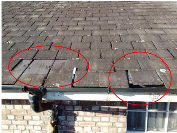
Evidence of Slate slippage on eaves course. As before described
