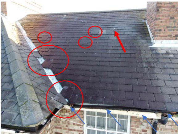
Evidence of loosening of slates due to wind damage, and possible vortex on leeward side of hip and leading to failure of fixings. All Guttering to be replaced.
