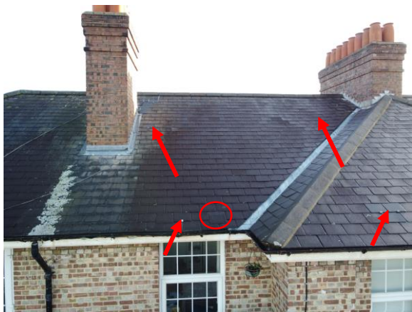
Slate identified as Penhryn ‘County’ Grade Natural Slate Evidence of slate slippage and previous attempts at repairs to localised slates.
