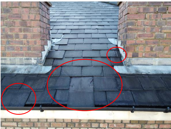
Slate not installed in compliance with BS5535:2018/BS8000 part 6. Recommend Abutment slates minimum 150mm so as not to compromise side-lap. Normally, all abutments should be taken from slate and half and we haven't seen any slate and a halves in use.
