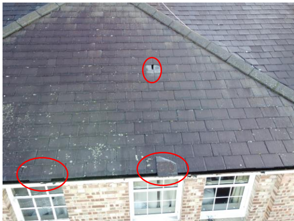
Insufficient or no fixings used to install roof covering. Under Eaves course of slates appears to have dislodged in places manifested by slate in gutter as shown.
