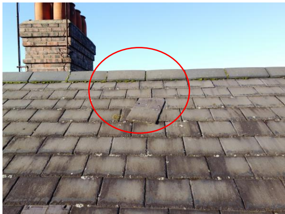
Integrity of ridge line starting to harbour moisture shown as green moss growth directly beneath ridge. Dark hue on circumference of slates is indicative of a higher level of moisture content/absorption. Further slate slippage.
