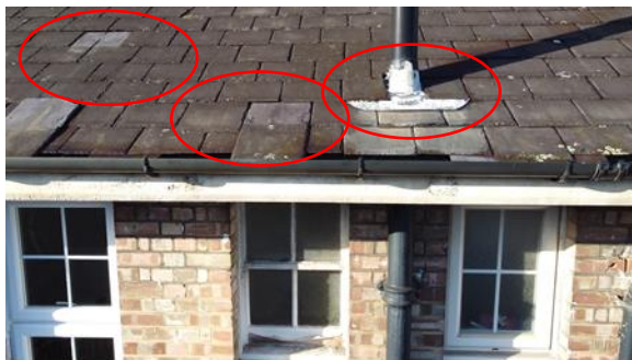
Failing lead slate to soil vent pipe and apply balloon Very strong evidence to support ageing of slates and tile slippage and nail sickness.
