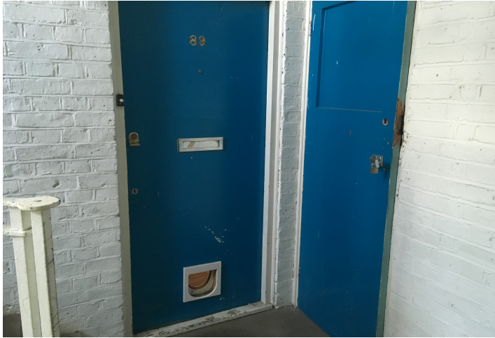
Fig 1; Internal fire doors with cat flaps should be removed and replaced with FD30s fire doors with intumescent strips, cold smoke seals and "Positive" self closing devices. Or installed with an Intumescent cat flap protector.
