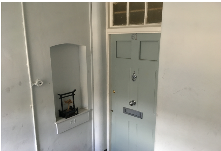
Fig 2; The internal windows and infill panels should be replaced with fire rated glass and frames. The original flat doors should be replaced with FD30s fire doors with intumescent strips, cold smoke seals and "Positive" self closing devices.
